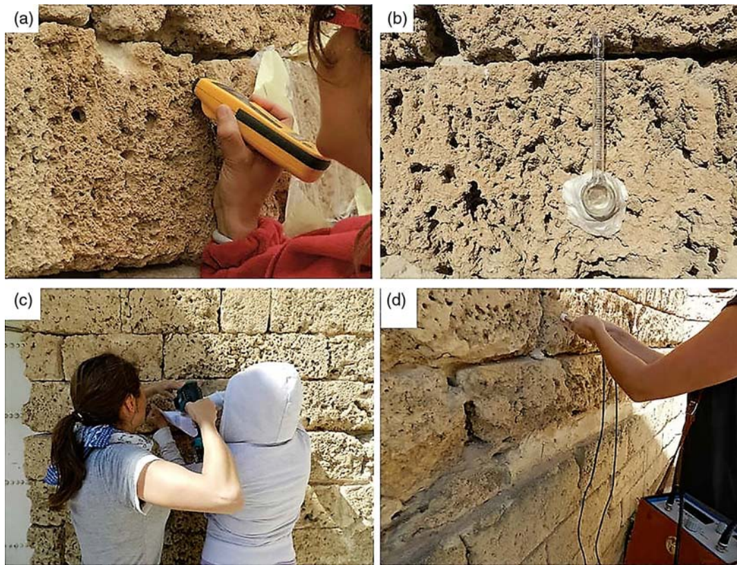
Fig. 3. On-site measurements with nondestructive techniques: (a) measurements of moisture content; (b) water absorption measurements by Karsten pipe; (c) sampling of stone powder by means of an electrical drill to perform further soluble salt measurements by ion chromatography analyses; (d) ultrasonic velocity ( V_p ) measurements
